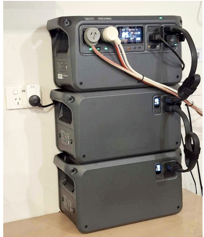
The left power outlet powers the video projector etc and the right outlet powers the modem and refrigerator/freezer. Image: John Rogers.
